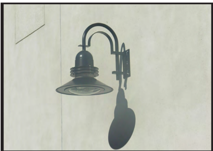
Where pole-mounted lights cannot be installed, a building-mounted light can provide illumination along an accessway and/or sidewalk.
