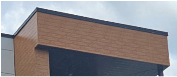
Cornices and parapets can be used as a cap and should be an accent element with materials and colors.
