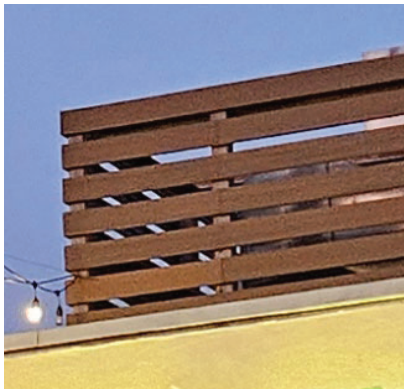
Screening can be used to create the required cap to Primary Facades & allow for code-compliant ventilation.
