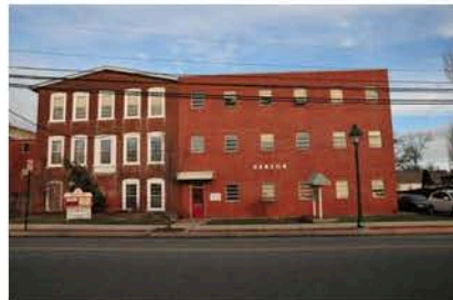
While the addition on the right retained the historic brick facade materials, the window dimension, proportions and spacing are inappropriate
