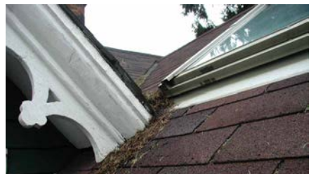
do allow clearances for drainage--this case is a little too tight
