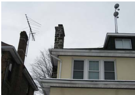
Satellite dishes & antennae create clutter and are water entry points.
