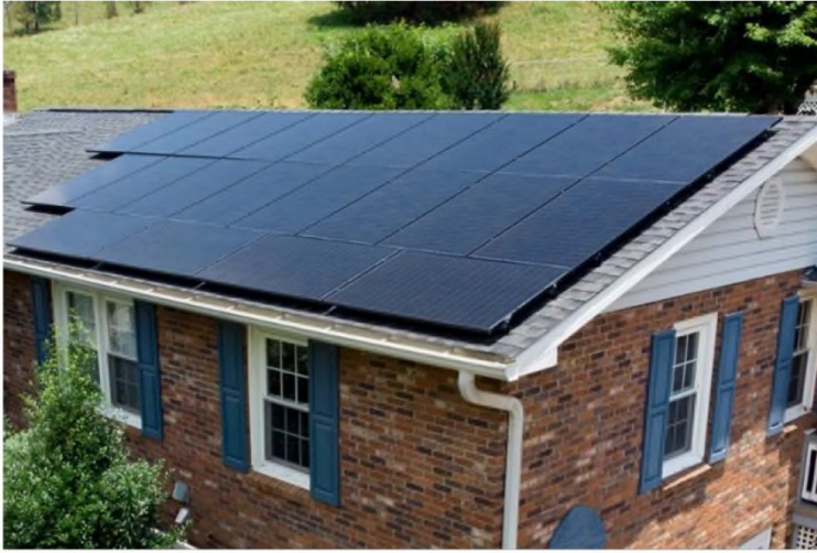
Residential installation, one story; photo courtesy of CNET, www.cnet.com
