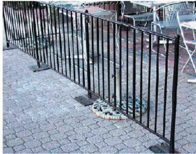
Figure 15. Acceptable pedestrian barrier.
