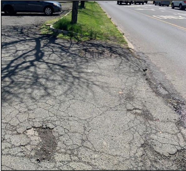
Picture 5 - Degraded macadam at the ingress on Terrill Road.
