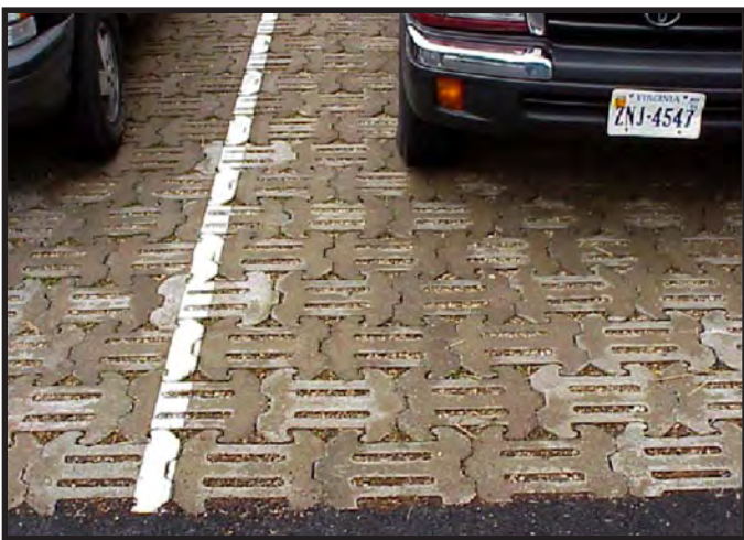
Parking area surfaced with porous Unit Pavers.
