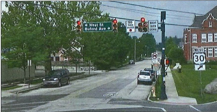
Facility on Existing Traffic Light
