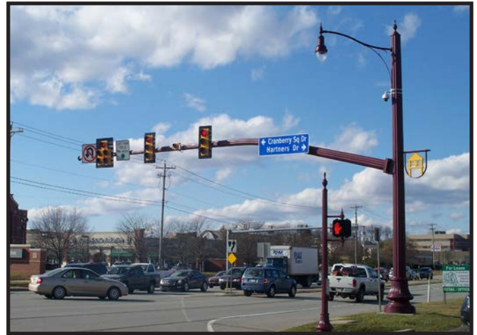
Traffic Signal and Poles, Route 19 at Cranberry Square Drive/ Hartners Drive, Cranberry Township
