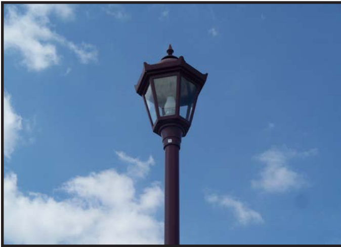
Street Light: Route 19 near Victory Drive, Cranberry Township
